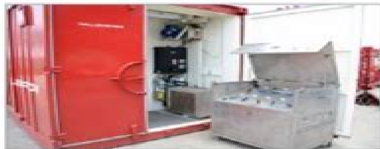
Chemical Injection Offshore Pumping Unit
